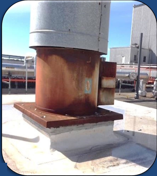
Boiler Stack Before MCU-100
