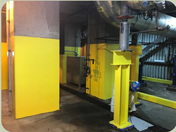
CM-15 High Solids Epoxy Mastic used on concrete and steel support beams.
